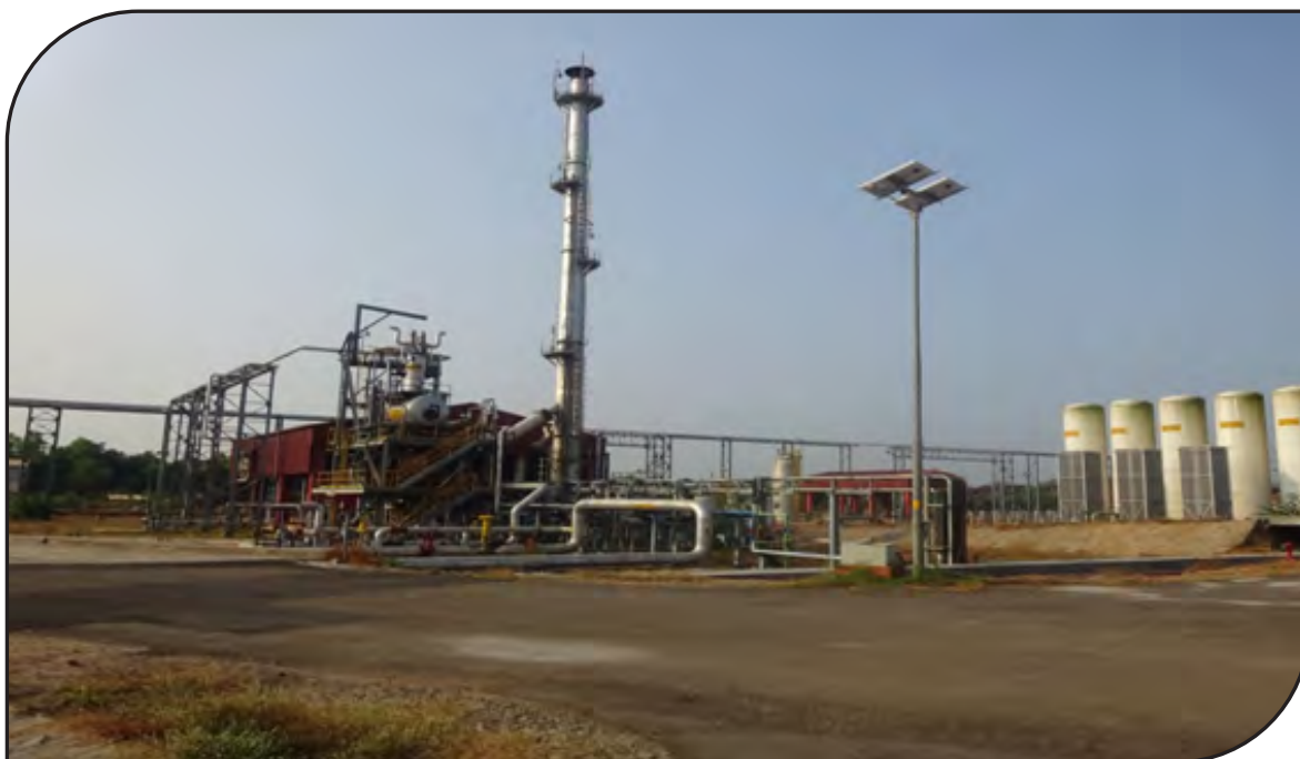
View of the aboveground facilities at Padur
