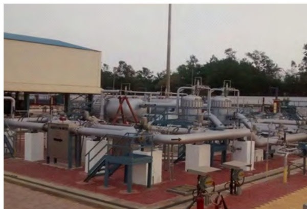
Jatni Station - Piping area
